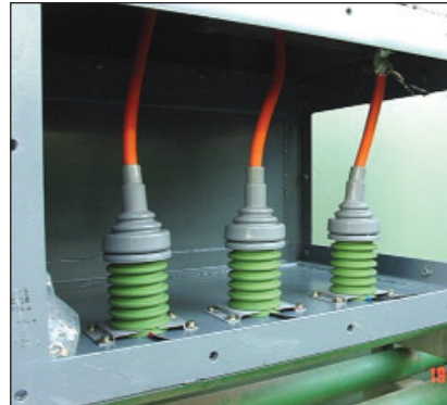
Installed Capacitive Coupler
